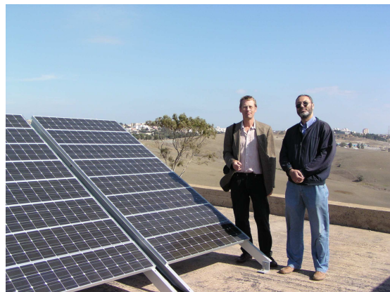
New 3 kWp grid connected PV installation of CREDEG in Alger
